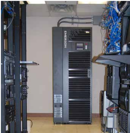
Liebert® eXM™ UPS with internal batteries and a slim maintenance bypass fits easily into the APH data center.
