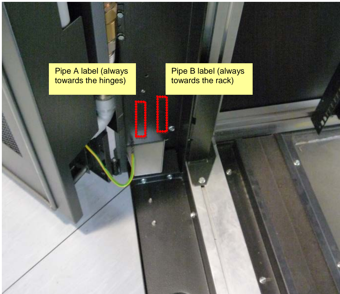
Figure 26 Pipe labels position
