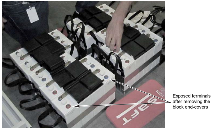
Figure 13.4 Removing Block-end covers to Expose Terminals
