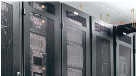
Integrated Racks And Cabinets
