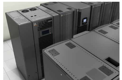
Liebert eXM adjacent to the wall
